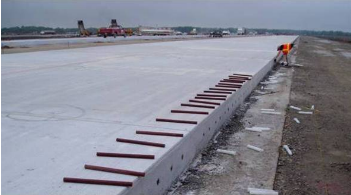
Figure 2. Test section for plastic sleeve at Hopkins International Airport in Cleveland, OH.
