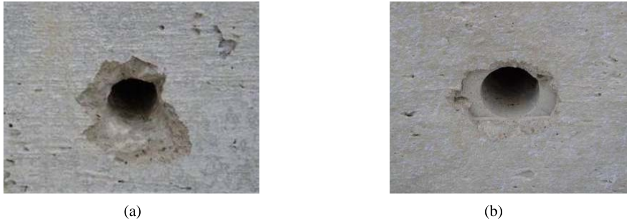
Figure 15. Quality of dowel support at the joint face: (a) typical spalling at the joint face of drilled holes; (b) smooth, formed hole produced by plastic sleeve.
